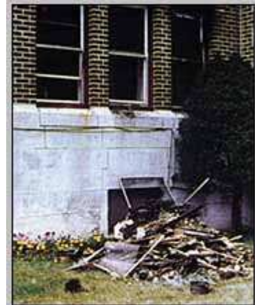
An all too common site? Fire debris, including plaster and lath walls and ceilings, is piled outside a building after a fire. An investigator arriving on this fire scene probably would be severely hampered in his ability to perform fire pattern analysis.
